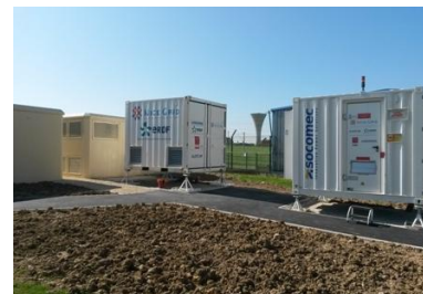
Figure 7 - Islanding testing system at Concept Grid
