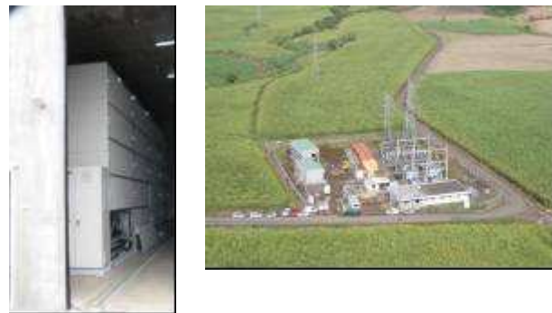
Fig.2: NaS battery module stacking. Internal view of the building. Substation view with the NaS battery and power conditioning system blocks.
