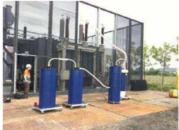
Fig. 1: from paper 166, after laying testing by a 250kV DAC system of a 6km long 150kV XLPE cable link
