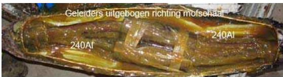
Fig. 11b: from paper 884, Field result: a similar joint as shown in previous Figure, which failed in service due to conductor extension.
