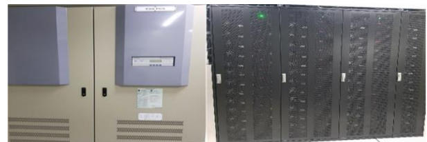
(a) 500kWh PCS and battery
