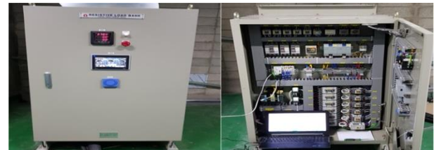
(b) 100kW load bank
