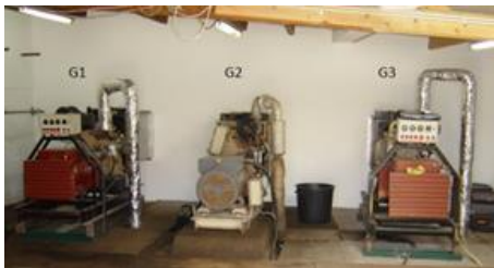
Figures 2: Group of generators
